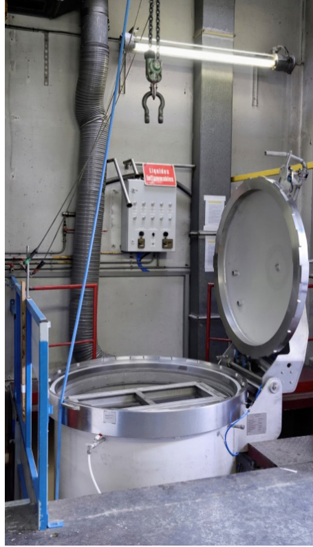
FIG. 26.4. Stainless steel resin impregnation tank.
